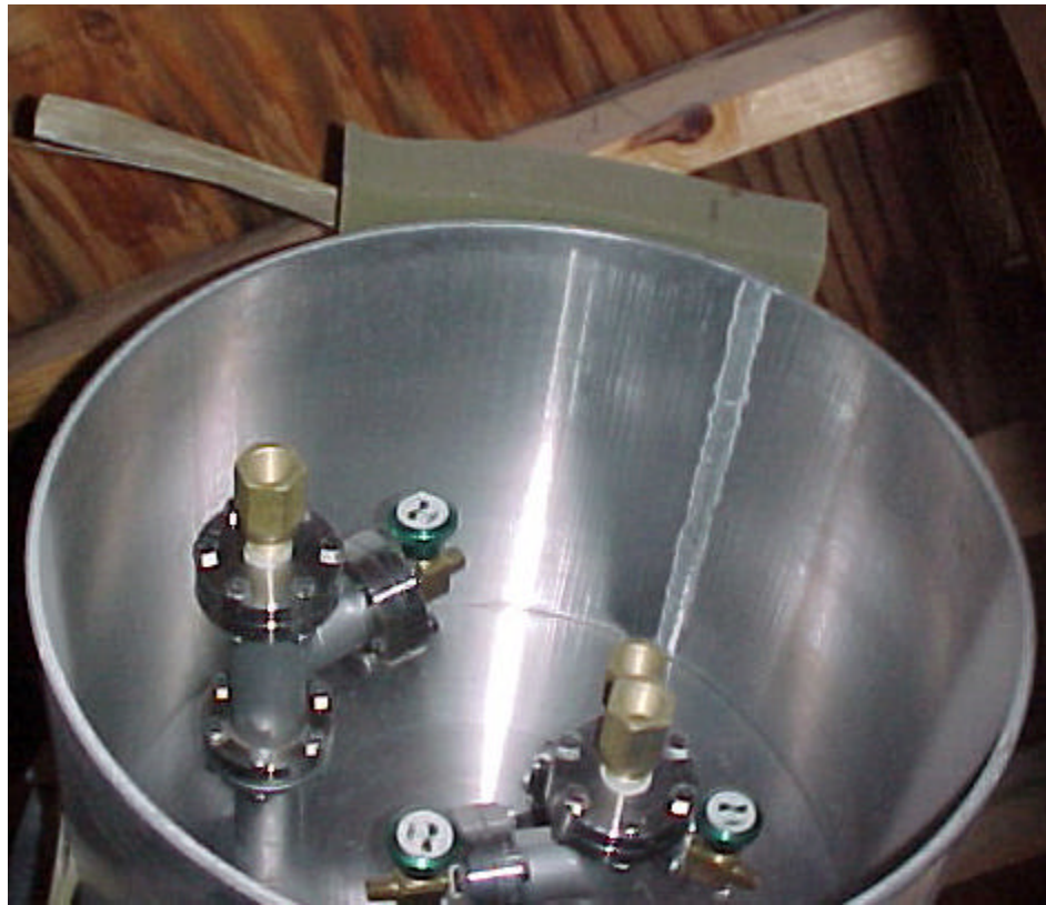
Figure 2: (top) The fourth coil valve assembly showing the pristine condition of the fourth coil service tower and (bottom) details of the valve assembly.
